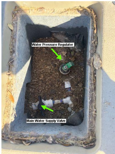
Main Water Supply Valve (Bottom) & Water Pressure Regulator (Top)
