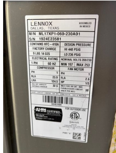
Condensing Unit Data Plate
