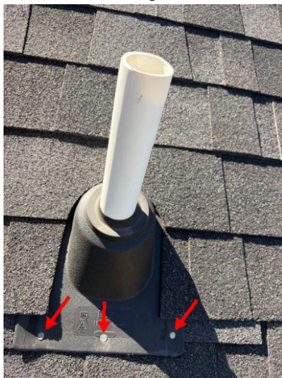
Exposed Roofing Nails
