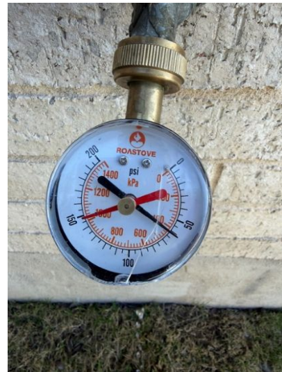
Static Water Pressure: 60 PSI
