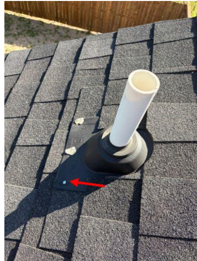
Exposed Roofing Nail
