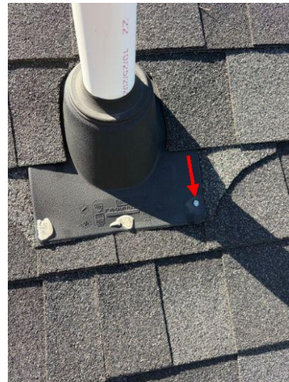
Exposed Roofing Nail
