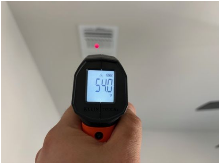
Cooling System Temperature Differential - 54.0°F at Supply Register
