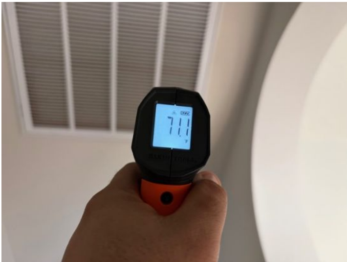
Cooling System Temperature Differential - 71.1°F at Return Register
