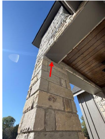
Gap between stone veneer cladding and soffit
