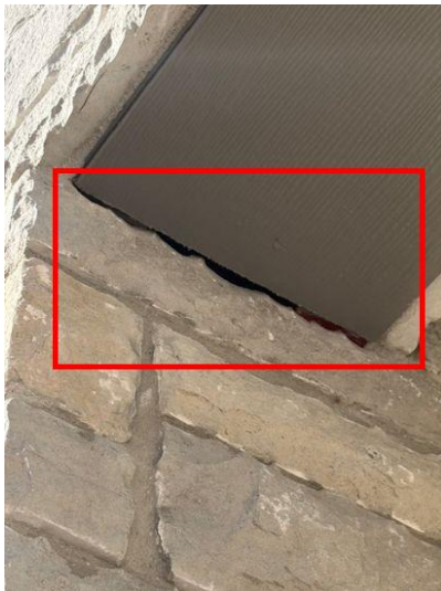
Gap between stone veneer cladding and soffit (Close-up)
