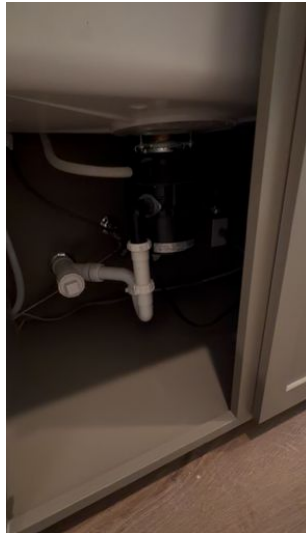
Kitchen Sink Drain - PVC
