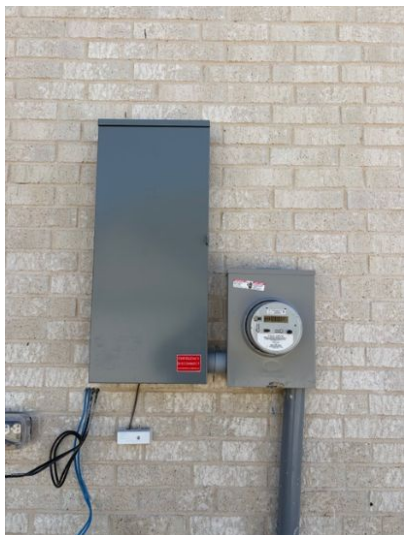
Electric Meter and Main Electric Panel
