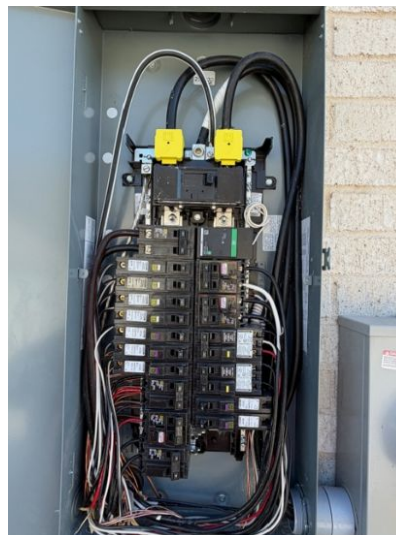
Main Electric Panel
