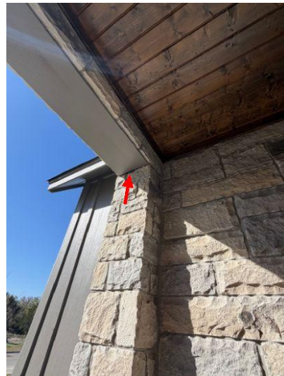
Gap between stone veneer cladding and soffit
