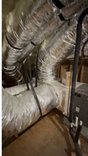
HVAC Duct System
