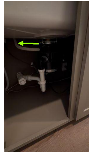
DW Drain Line High Loop
