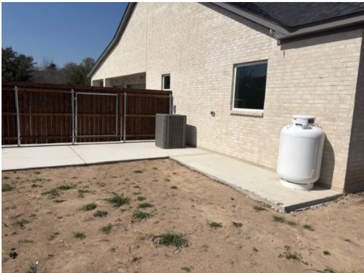
120-Gal Propane Tank
