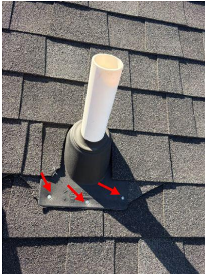
Exposed Roofing Nails
