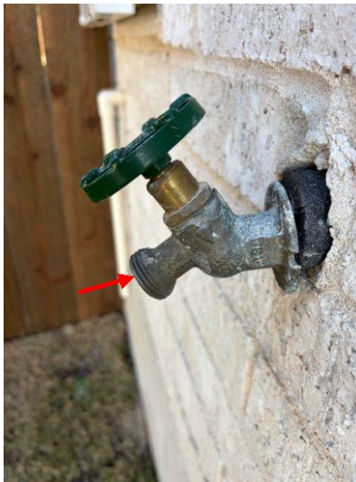
Missing Anti-siphon Device
